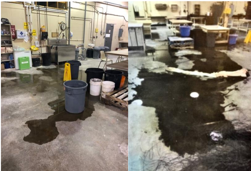
Jane Street Studio leak issues
